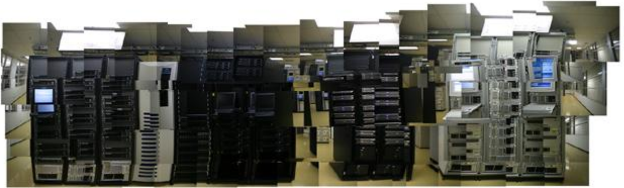
EEC control center montage
